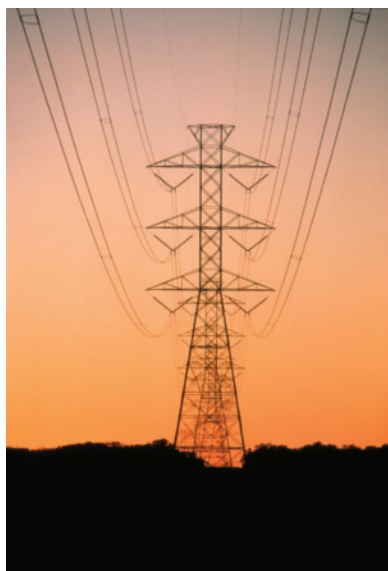
Figure 1 Electricity travels from the power plant to your home along transmission lines.
